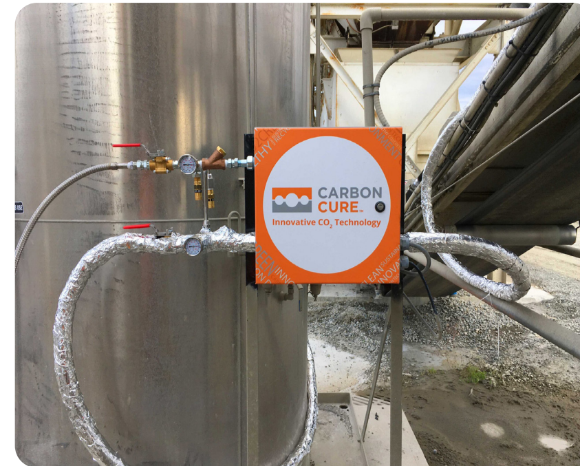
Figure 58. CarbonCure Concrete Valve Box
