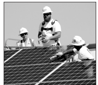
Only a few solar panels still need to be installed. (Photo by Jeanne Baron)
