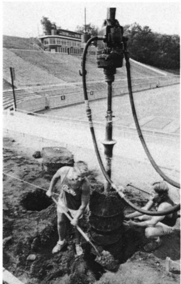
STADIUM SEATING SWELLS — Workers from Engineered Stadium Systems of Three Rivers are busy this summer installing an additional 5,200 seats in Waldo Stadium. The stadium improvements are needed to preserve the Mid-American Conference's National Collegiate Athletic Conference Division I-A status in football. The $200,000 project is being funded by a low-interest loan from the league. In addition to the 2,500 new seats being installed here in the northeast end zone, 2,700 portable bleacher seats will be put up in the southeast hill area on both sides of the press box. When completed at the end of the summer, the new seating will raise Waldo Stadium's capacity to more than 30,000.
