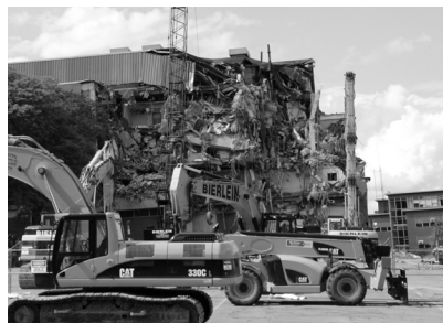
Demolition of the new wing of McCracken Hall with the Seibert Administration Building in the background (Photo by Jeanne Baron)
