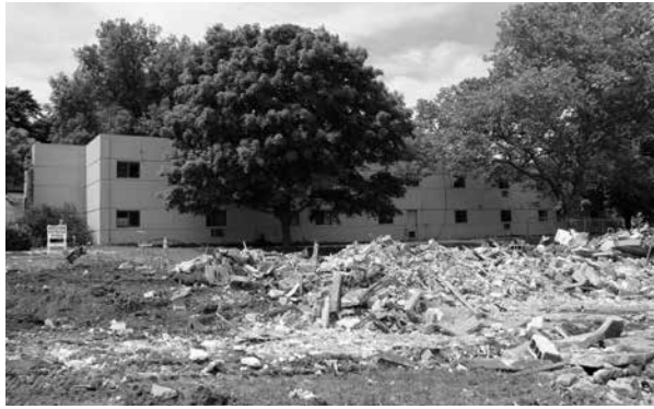
All 16 buildings in the Elmwood Apartments complex have now been razed. (Photo by Jeanne Baron)
