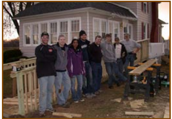
Some of the volunteers pictured next to the nearly completed wheelchair ramp.
